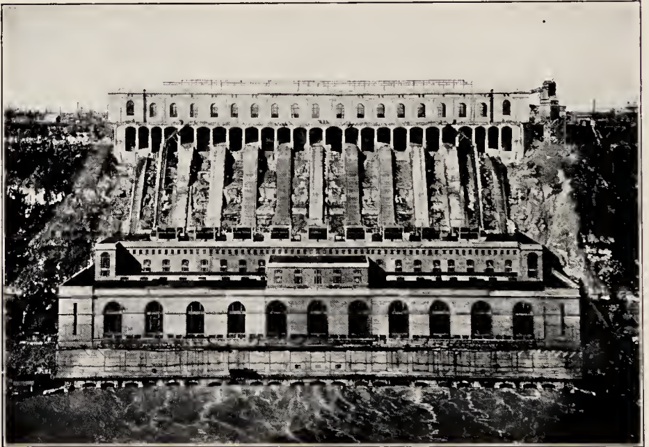
A bucket of water dropped down this cliff to the Niagara River would strike with the force of thirty horse-power. Imagine 20,000 buckets dropped every second and you have the capacity of this 600,000 horse-power station.
